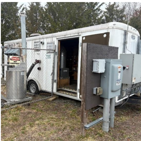
Photo 1: Area A Site LF042 AS/SVE system.
