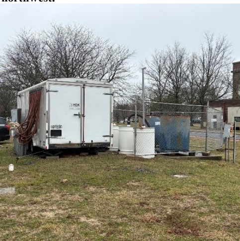
Photo 9: Area B Site TT013 AS/SVE system.
