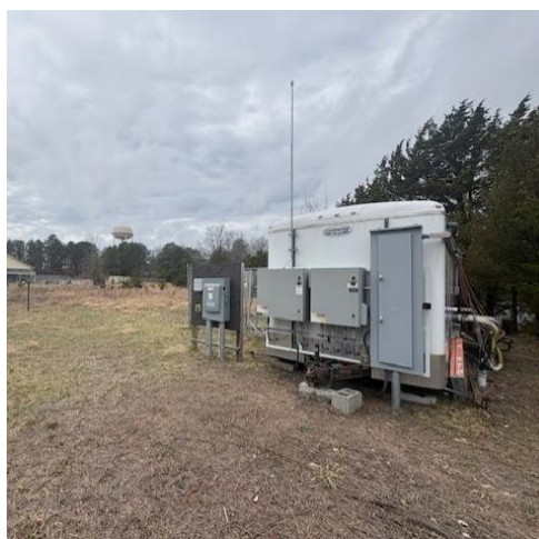
Photo 4: Area A Site LF042 AS/SVE system.
