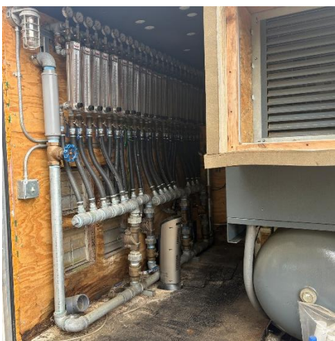
Photo 3: Area A Site LF042 AS/SVE system.
