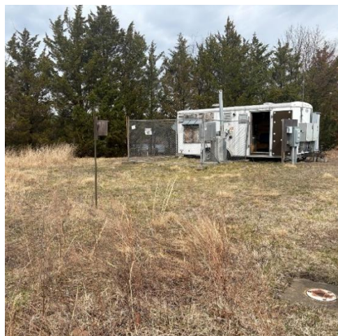
Photo 2: Area A Site LF042 AS/SVE system.
