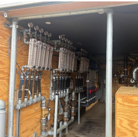
Photo 11: Area B Site TT013 AS/SVE system.
